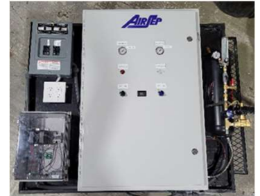
On-Site Oxygen Generator
