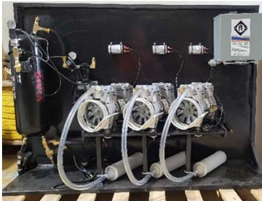
Compressed Air Supply
